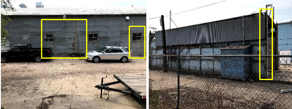
Figure 2. Deteriorated Exterior Finishes and Ancillary Structures
