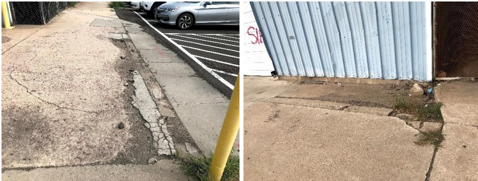
Figure 5. Cracked or Uneven Surfaces for Pedestrians
