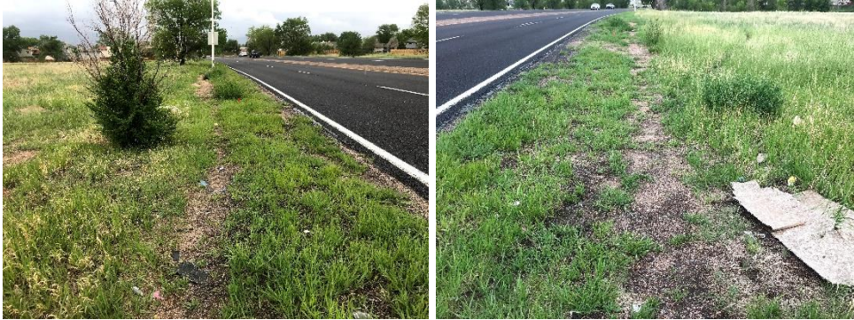
Figure 2. Lack of Sidewalks
